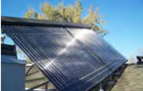
Evacuated tube solar water array
