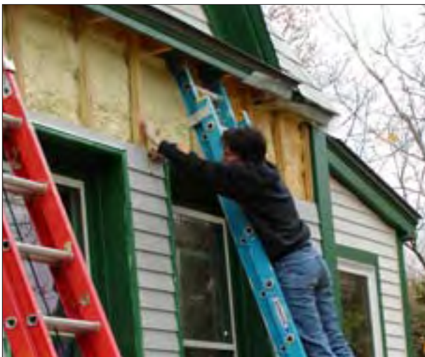
EA45 Exterior Wall Air Sealed and Insulated with Spray Foam; Reclad (note exterior jamb extensions furring)
