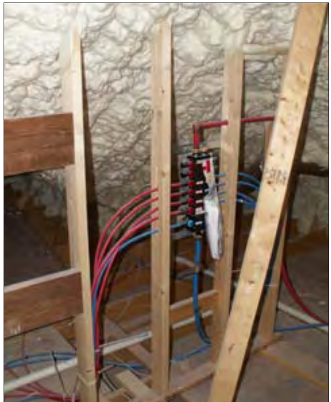
EA77 PEX Plumbing for Efficient Distribution of Hot Water
