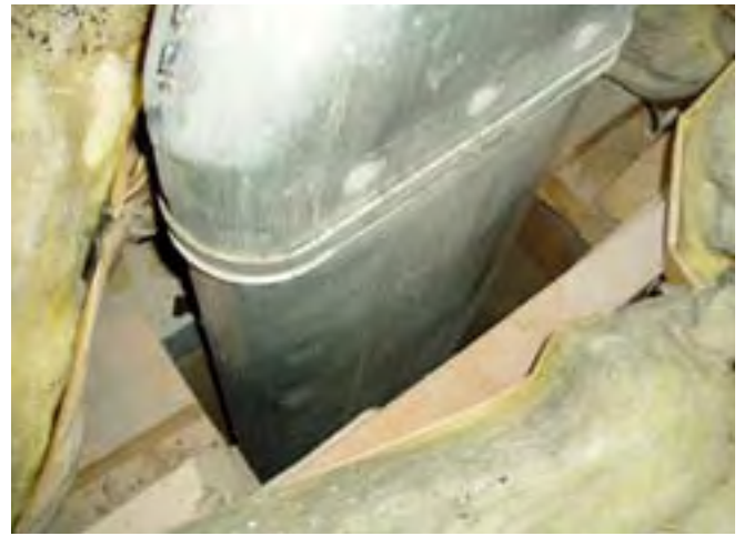
EA54 Thermal Bypass: Duct Chase
