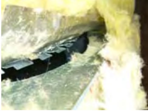
Before – duct leakage
