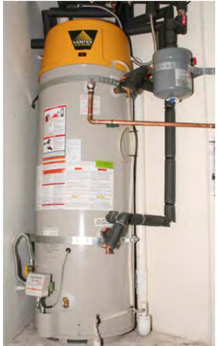
After – power vented high-efficiency water heater
