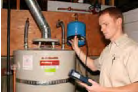
Home performance audit: testing water heater draft
