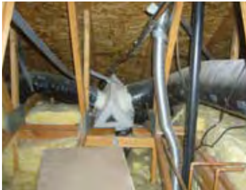
Before – bad ducting
