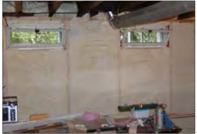
EA47 Furred Out and Spray Foamed Basement Walls (vapor-permeable polyurethane)
